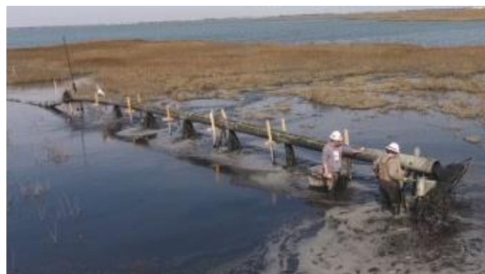
Sediment Distribution Pipe demo on Sturgeon Island March 2020 as part of the Innovative Sediment Distribution Pipe for Targeted Placement project in Philadelphia District's Seven Mile Island Innovation Lab in New Jersey.
